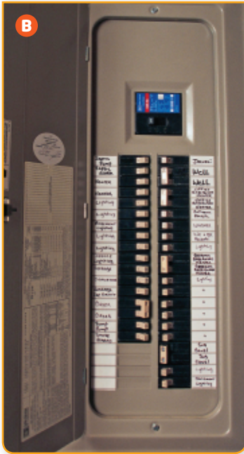
Figure 12.4 A All electrical energy use is metered. B In a typical home, the meter is in series with the wires from the street transformer and a distribution panel like the one shown here.
