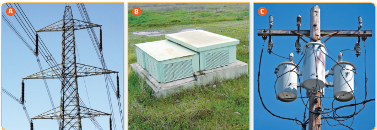
Figure 12.3 A The thin wires at the top of the tower are grounded to help protect the system from lightning strikes. The high voltage is between adjacent wires, not between the ends of a single wire. Insulators stop adjacent wires from touching. B Transformers step down the voltage before a line is connected to the meter at your home. In towns and cities, wiring is underground and step-down transformers are often inside green boxes. C In rural areas, cylindrical pole transformers are the norm.
